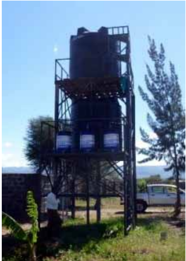
Photograph courtesy of EAWAG Figure 13. The bone char defluoridation plant, of the Catholic Diocese of Nakuru, CDN, Kenya.
